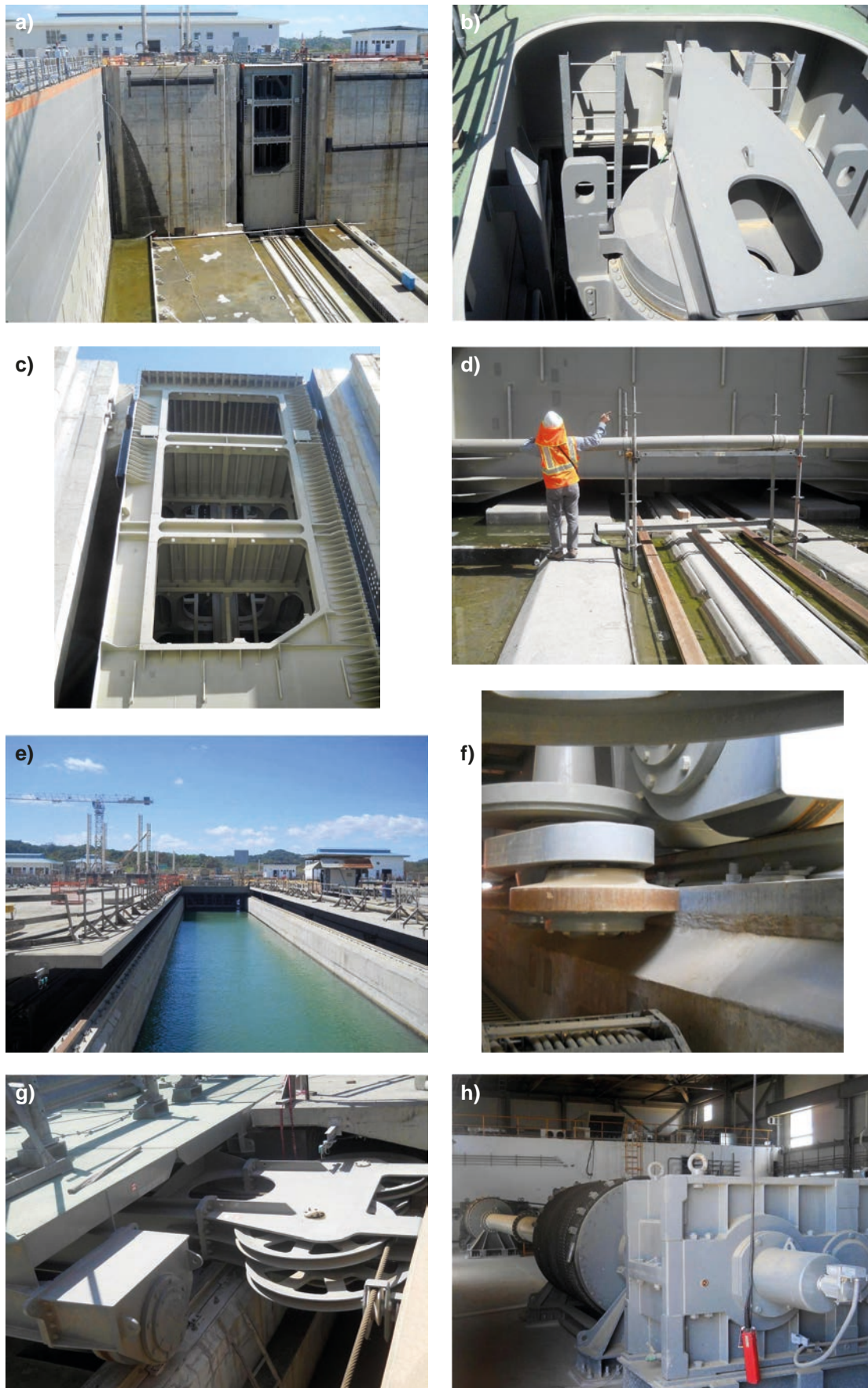
Fig. 12. Gates of new Panama Canal Locks during commissioning, photos I. Hermans
