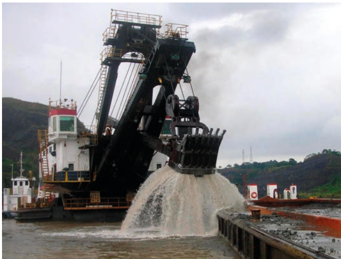
Fig. 4. Backhoe dredger Rialto M. Christensen at work in Culebra Cut (photo P. Meesen)
